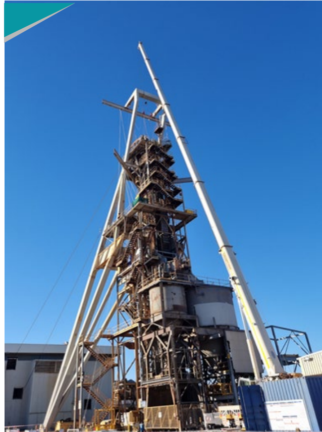
AusGroup - MAS Head frame remediation project via Rope Access at a Nickel mine
